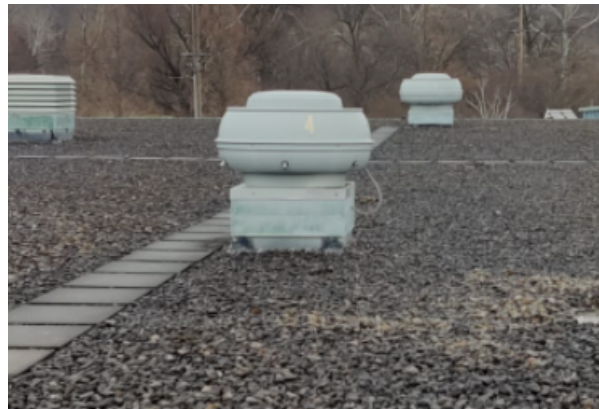
Figure 4.3: Example Vent on TCAT Roof
